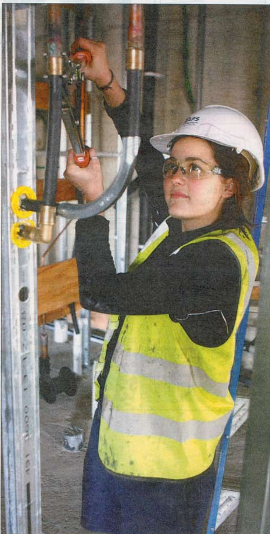
IN SAFE HANDS: Apprentice plumber Carly Gerrard at work at the University of Adelaide site yesterday. Picture: JO-ANNA ROBINSON
